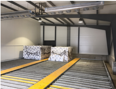
Inside one of the temperature-controlled chambers of WFS' new pharma facility in Copenhagen.
